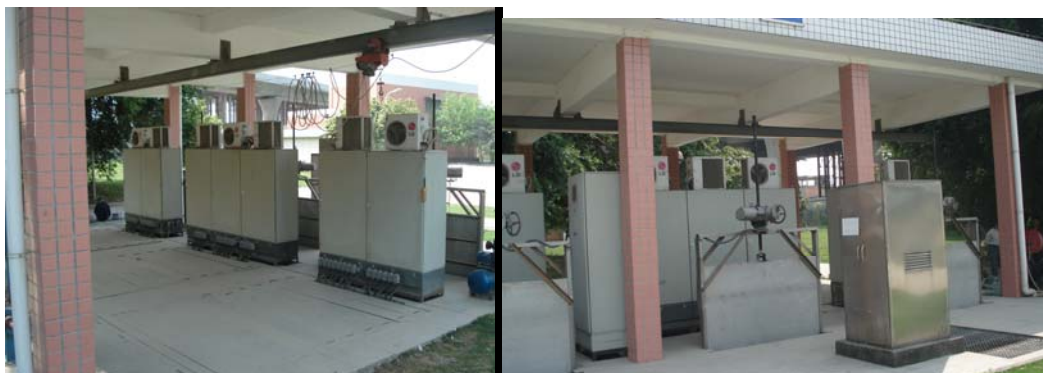
Newland channel system with 380 UV lamps at Fuzhou Wastewater Treatment Plant.
