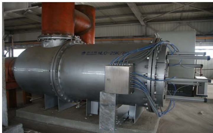
Newland closed reactor UV system at Beijing Miyun Water Purification Treatment Plant 50,000 m3/day
