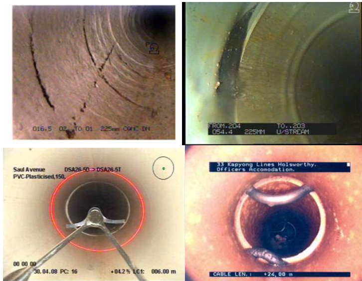
Figure 4: Examples of defects in new sewer and stormwater installations
