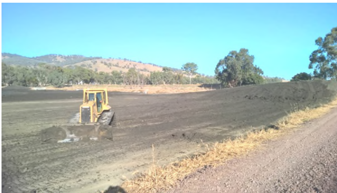
Figure 1: West Wodonga WWTP Drying Pans.
