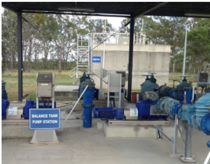
Figure 3: Raw Sewage Balance Tank (RSBT) Pump Station in the foreground with Flow splitter in the background – Burpengary East STP.
