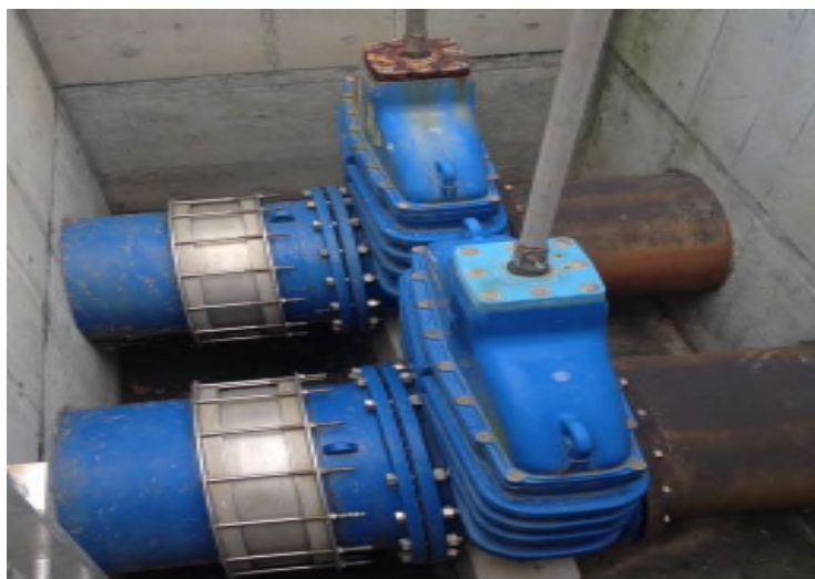
Figure 4: Raw Sewage Balance Tank (RSBT) Isolation Valves – Burpengary East.
