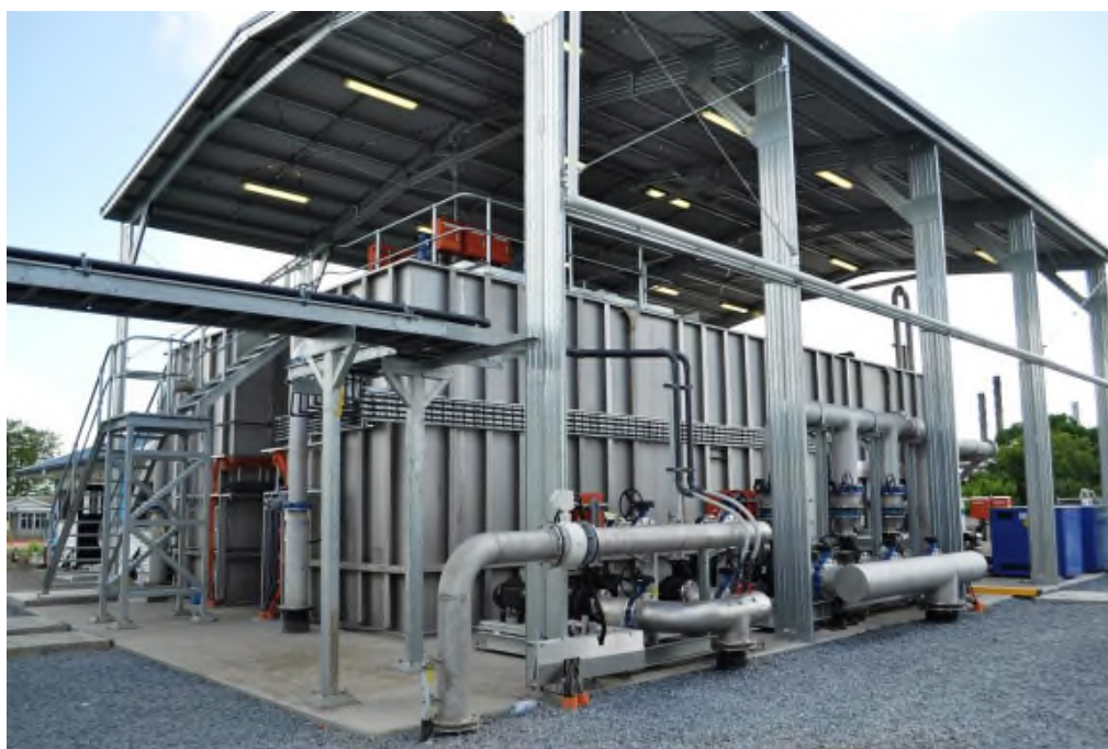
Figure 2: Marian Water Treatment Plant.
