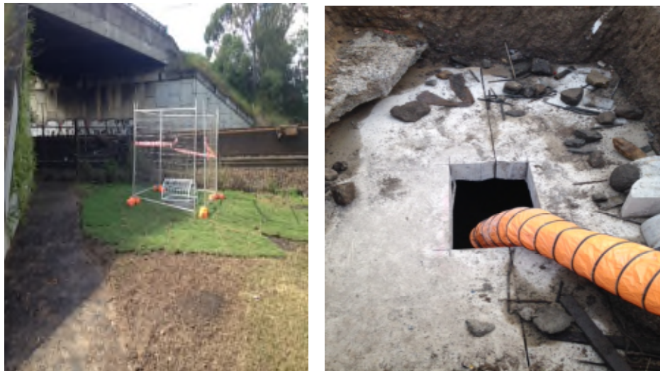
Figure 7: An Access Hole Cut in the Culvert Roof During Cleaning was Converted to a Field Drain for Future Access.
