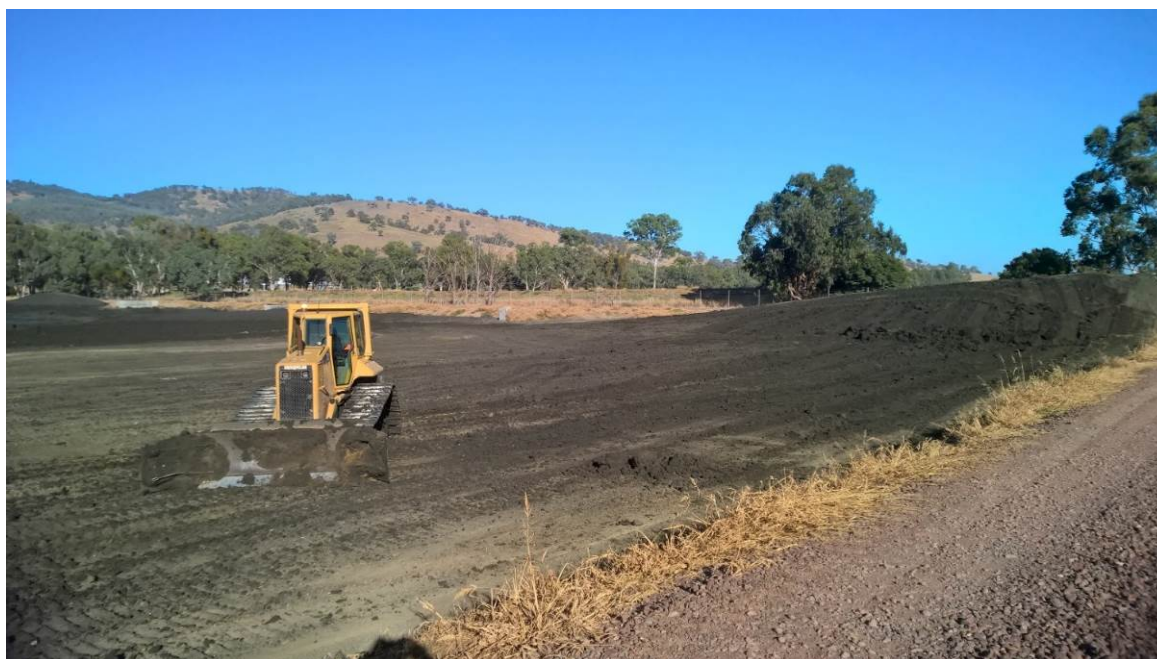
Figure 1: West Wodonga WWTP drying pans
