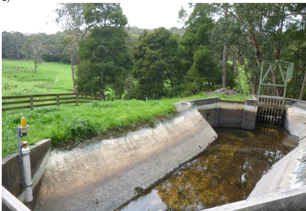
Figure 4: Old King's Syphon Trash Rack & Blok-aid
