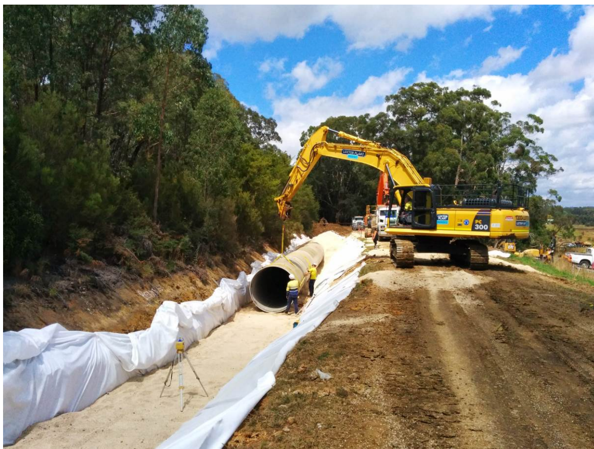
Figure 5: Piping of the WBIC
