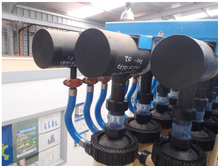
Figure 4: Upper Membrane Manifold where Level Switch will be Located
