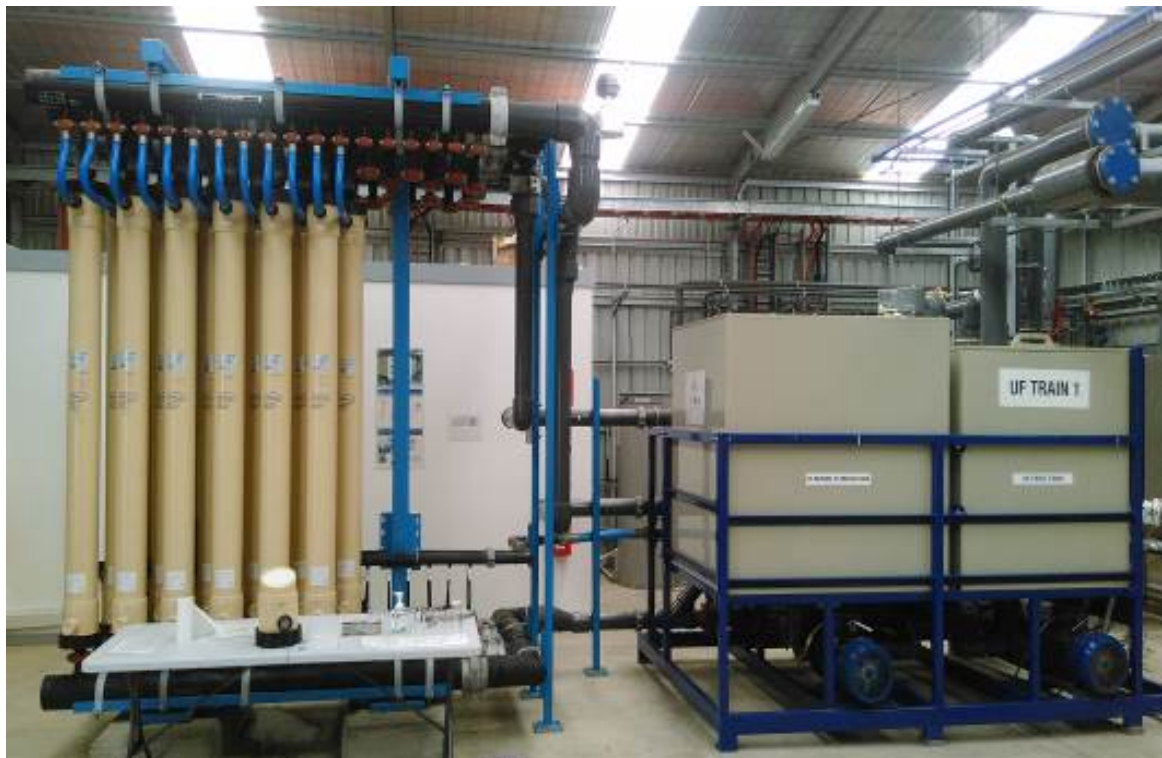
Figure 3: Side View of Membrane Modules and Feed Water Tank
