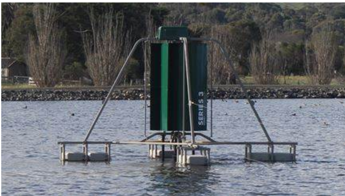
Figure 2: Series 3 Wind Mixer Installed in Wastewater Lagoon
