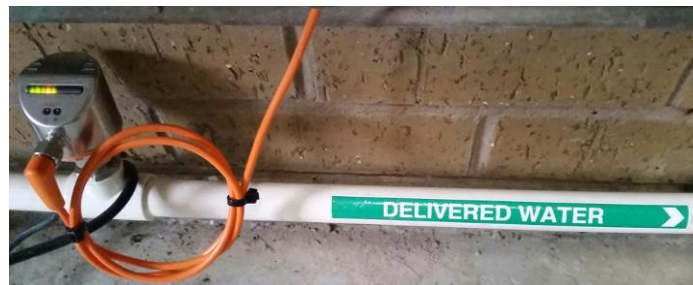
Figure 3: A Flow Sensor on a Sample Water Pipe.
