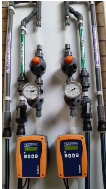
Figure 4: A Sodium Hypochlorite dosing installation showing the chemical flow meters, backpressure valves and carry water pipe work.
