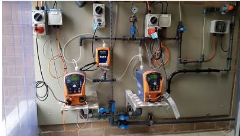
Figure 2: A Sodium Hypochlorite dosing system incorporating dosing pumps, flow meter, backpressure valve, pressure gauge, carrier water supply and check valves.
