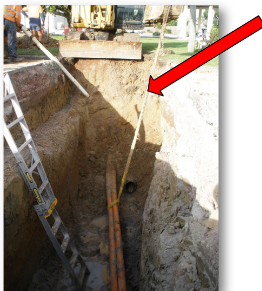
Figure 2: The Excavation – Showing Conduit, Pipe and Location of Wall Collapse
