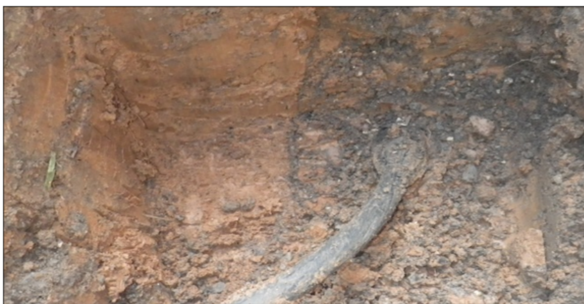
Figure 4: Original Repair - Rural Grade Poly Pipe
