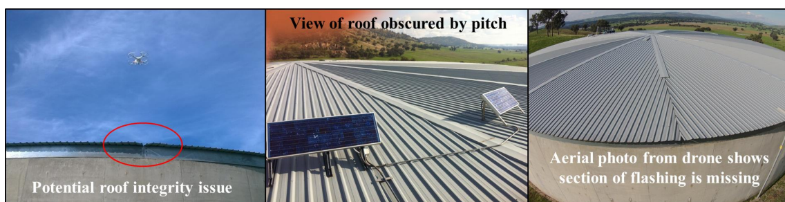
Figure 2: Photos Taken from Ground, Roof and Air of Damaged Clear Water Storage Roof
