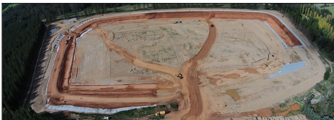
Figure 5: Photo Taken by the Drone of a 520 ML Off-river Water Storage Under Construction at Bright.
