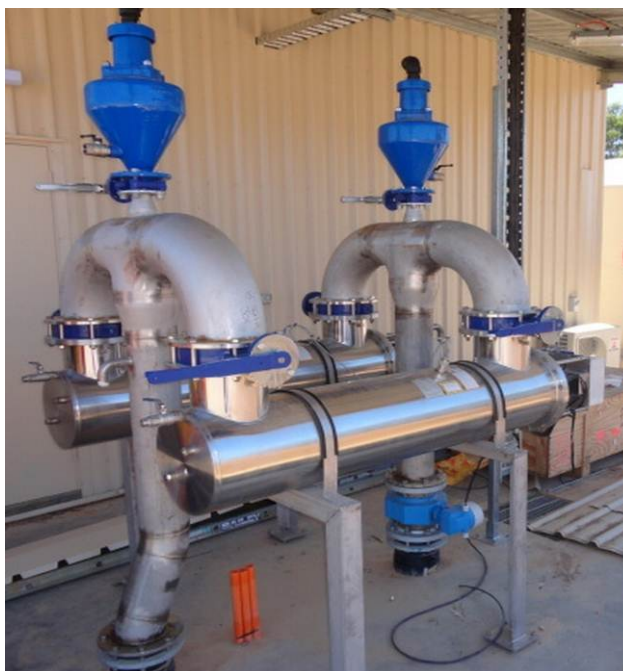
Figure 6: UV disinfection unit
