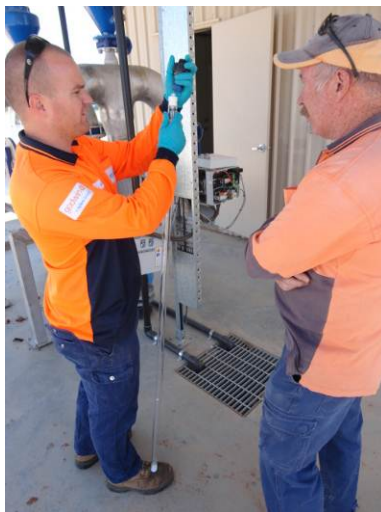
Figure 2: The operators inspecting an Ultra Violet lamp
