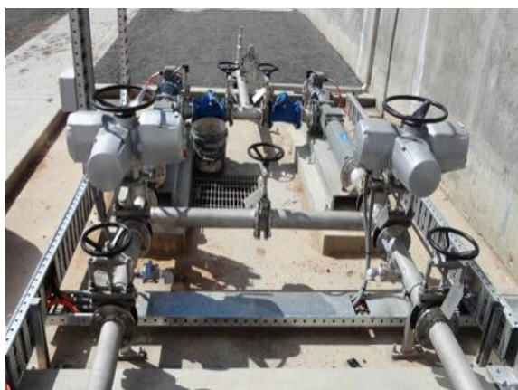
Figure 4: The WAS pumps at Warracknabeal
