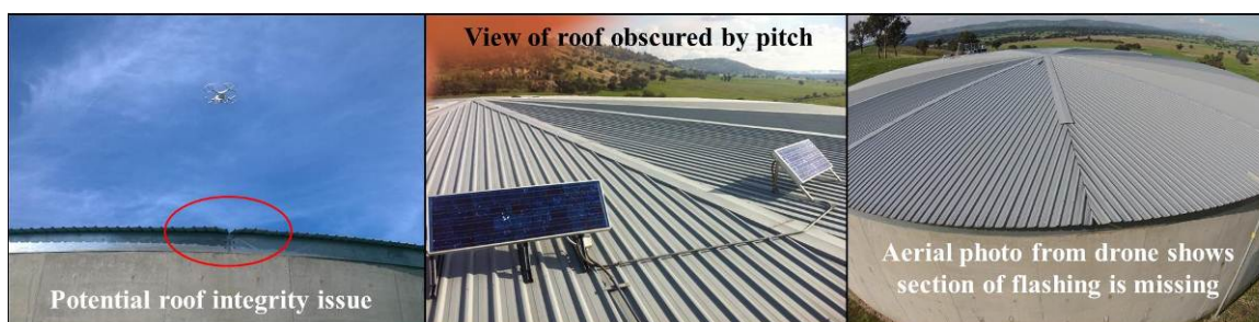
Figure 2: Photos taken from ground, roof and air of damaged clear water storage roof.
