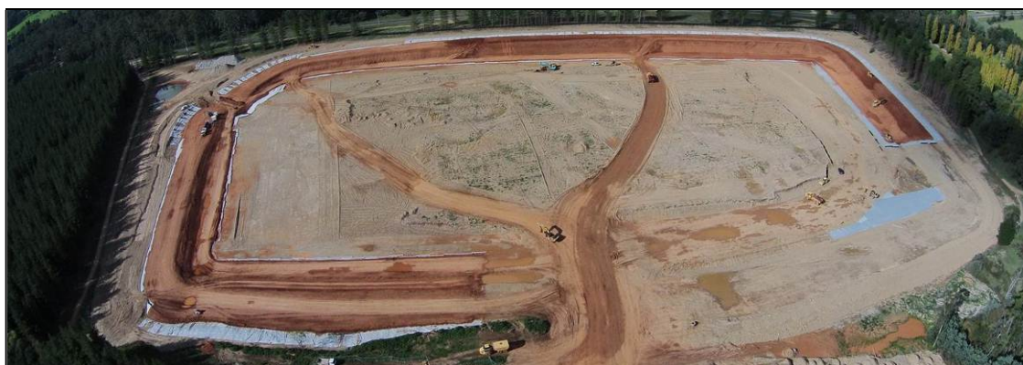
Figure 5: Photo taken by the drone of a 520 ML off-river water storage under construction at Bright.
