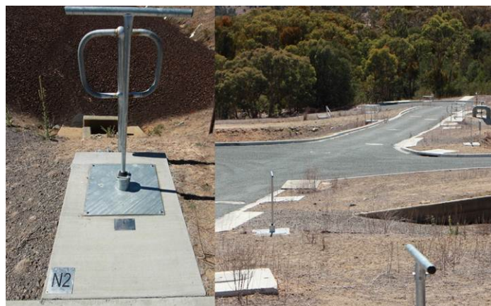
Figure 2: New Drying Bed Inlet Valves. Left showing the new valves with labels the right showing a row of closed inlet valves.
