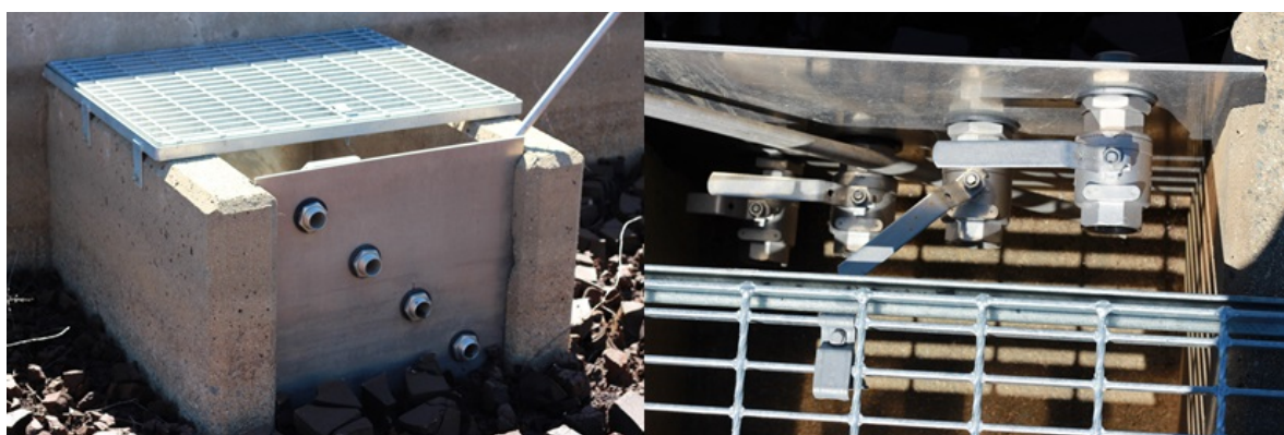
Figure 4: The new Drying Bed Decanting Weir Boards showing the 4 valves at differing levels.
