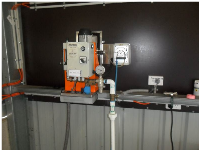
Figure 2: TOMAL liquid polymer dosing system
