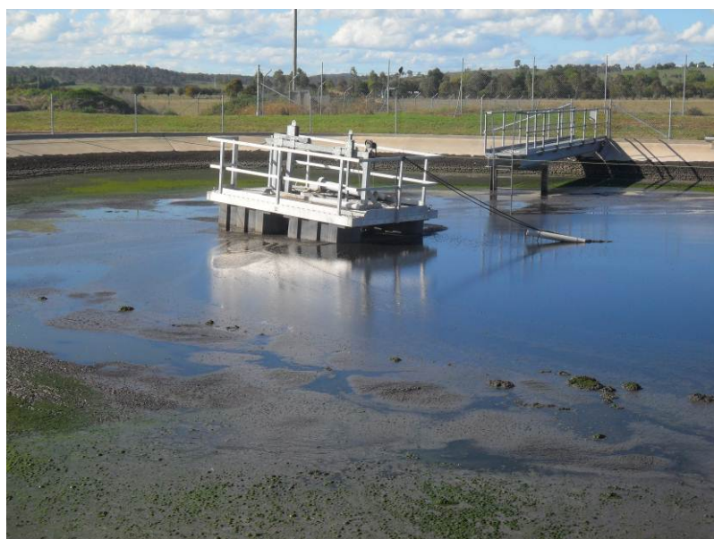
Figure 3: Pontoon mixing pump with variable speed drive
