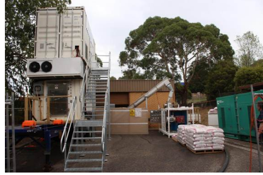
Figure 6: Ice Making Plant
