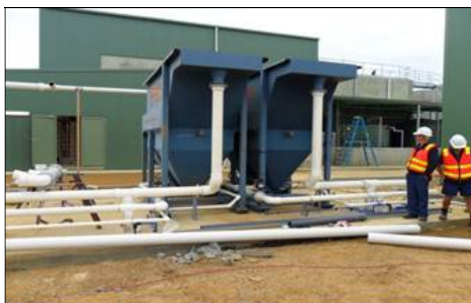
Figure 3: Lamella clarifiers used to process washwater at Woodglen WTP
