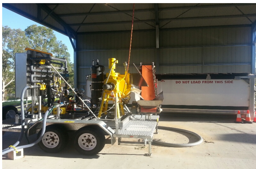
Figure 1: New Dewatering Building system at Jimboomba.
