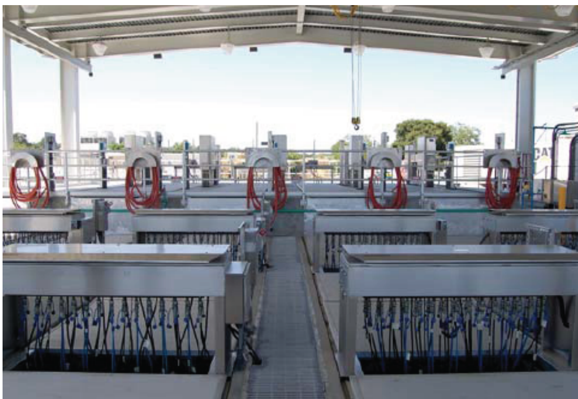
Figure 2: The plant's five effluent channels are treated with a Trojan UV3000Plus™ disinfection system. Each channel has four banks of low-pressure, high intensity amalgam lamps.
