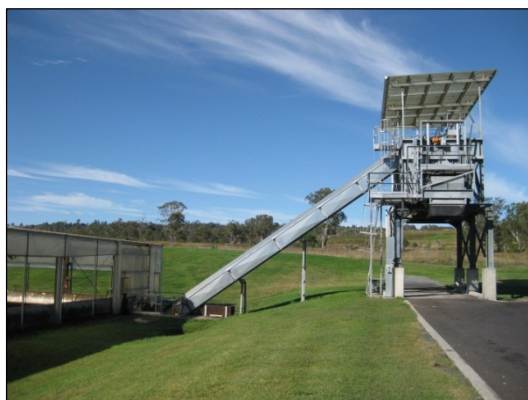
Figure 5: Conveyor to dry Hopper
