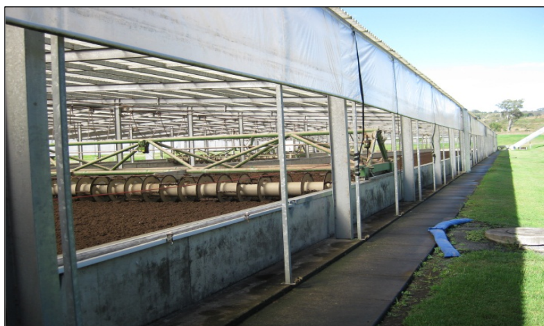
Figure 3: Solar Drying Hall Curtains
