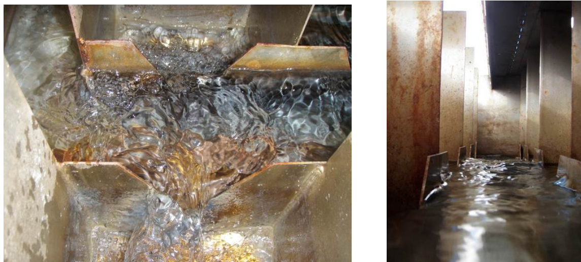
Figures 3 & 4: Polymer Splitter box V notches and turbulence.
