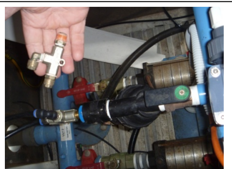
This an inline valve which often fails at Maroon Dam WTP
