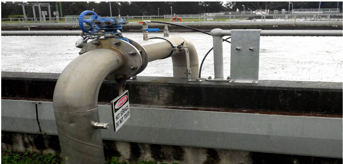
Figure 4: Diffuser maintenance fittings
