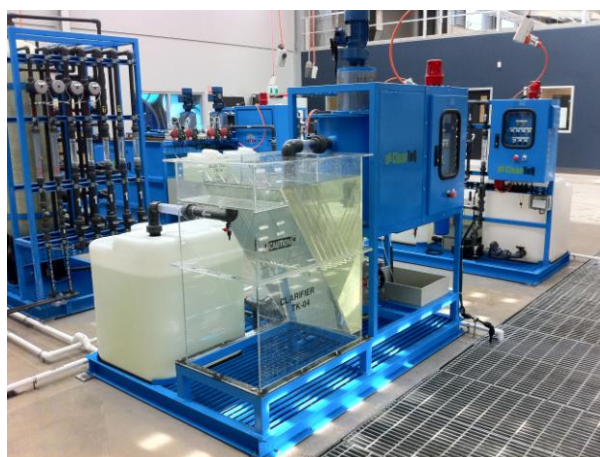
Figure 4: Clarifier, Flocculation and Coagulant Module
