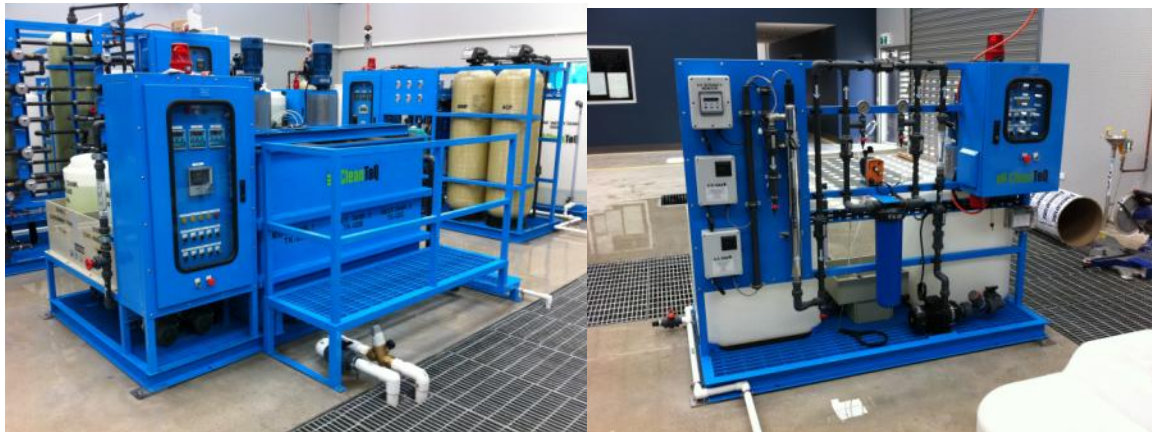
Figure 8: Effluent Neutralization System & Chlorine Dosing System with UV Sterilization
