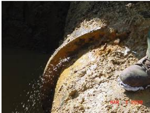
Figure 5: Small Leak in 900mm Pipe
