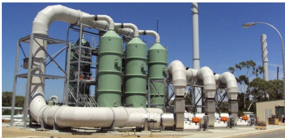
Figure 5: The Biological OCS as installed at the Beenyup WWTP, W.A.
