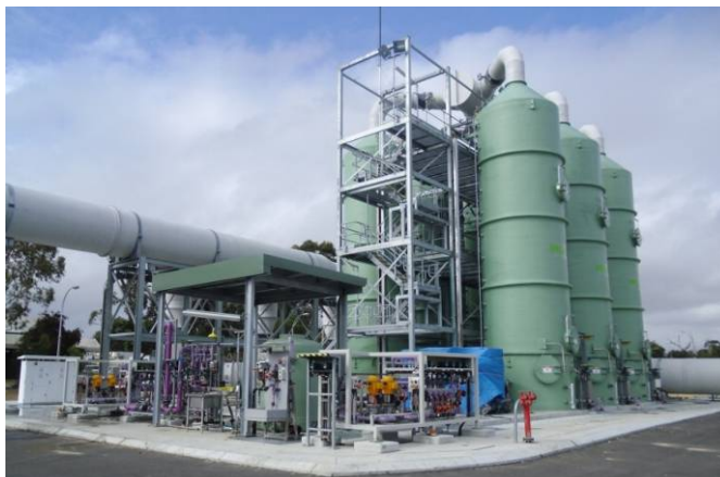
Figure 1: The Biological OCS at the Beenyup WWTP, W.A.
