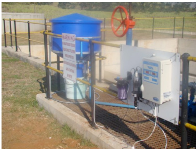
Figure 4: Feeder, pH /Redox controller adjacent to the chlorine contact tank
