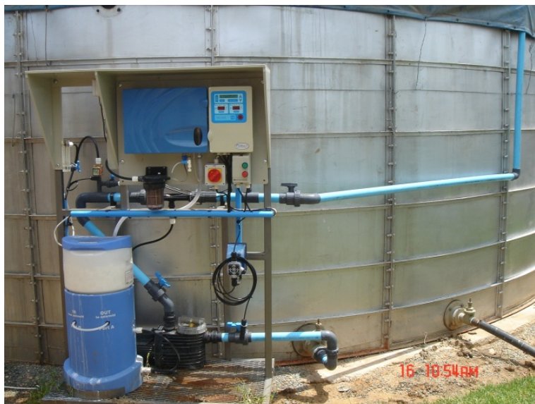
Figure 7: Dosing CH at a small reservoir – feeder, pumps and analyzer housed in a skid unit
