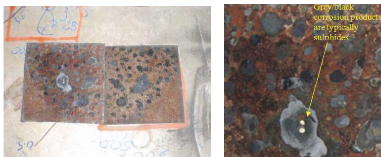
Figure 1: Under floor corrosion examples
