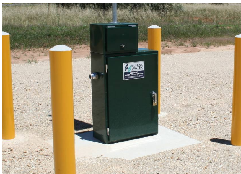
Figure 4: The installed bulk water filling station
