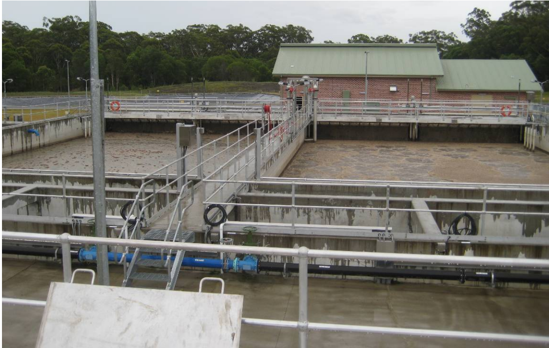
Figure 2: Intermittently Decanted Extended Aeration Tanks
