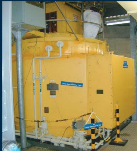
Pump Station, Yering Gorge
