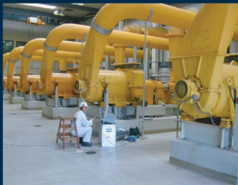
Water Treatment Plant, Chelsea
