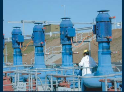
Pump Station, Werribee
