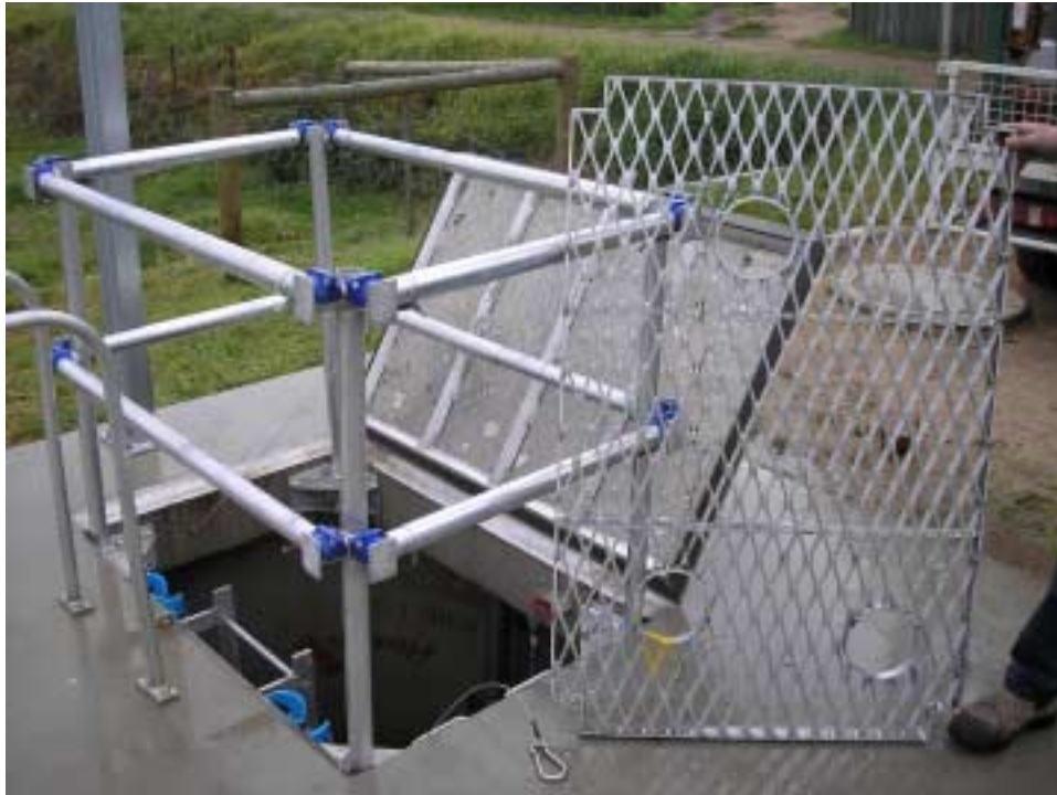
Figure 4: Fully Installed Handrail System with Grate Removed
