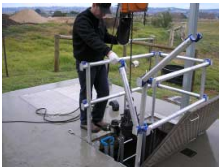
Figure 6: Practical Use of the Handrail System – Removing Pump
