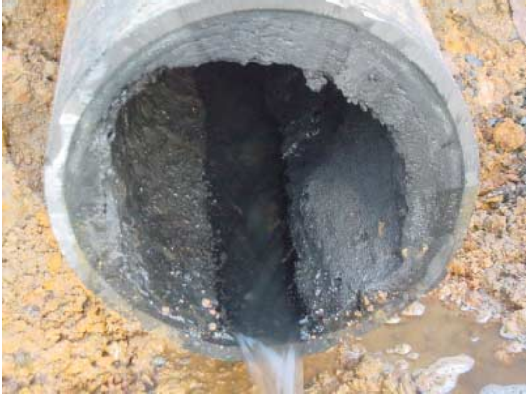
Figure 2: Sludge Build-up in Sewer
