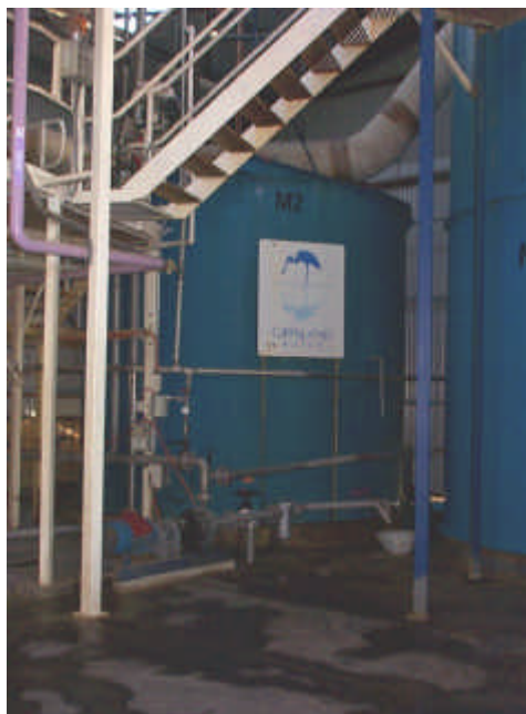
Figure 2: Gippsland Water's bulk alum quarantine tank at the Aluminates factory site
