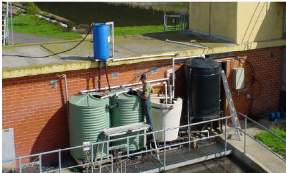
Figure 2: Pilot Plant located at Ballarat North Wastewater Treatment Plant
