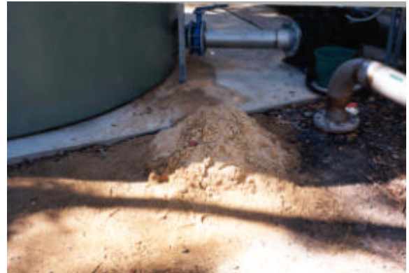
Figure 10: Result of a broken under drain nozzle. Sand entered the backwash tank and was redistributed to other filters. This required significant work to remove the sand and resulted in other filter rebuilds.
