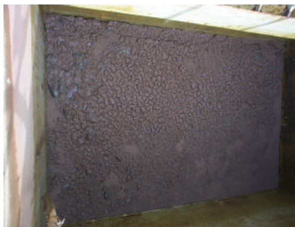
Figure 3: A 50mm Sludge layer that clearly shows cracking and shrinkage
