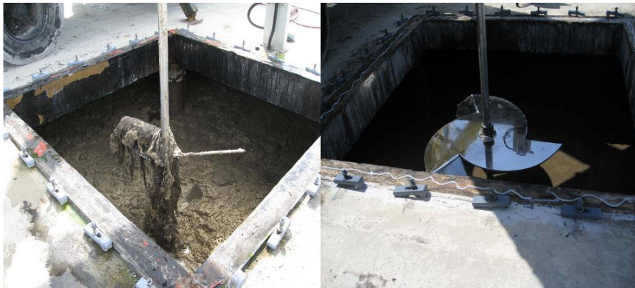
Figures 4 & 5: The first Clean-Edge impeller installed in STP in USA
