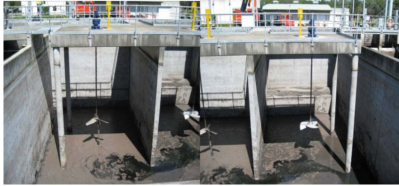
Figures 6 & 7: The new impellers at the Banora Point plant
