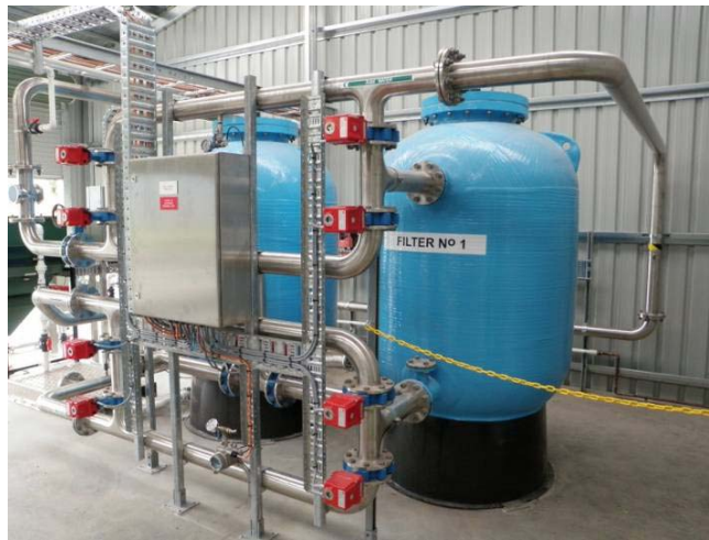
Figure 1: WTP filter cells with manifolds
