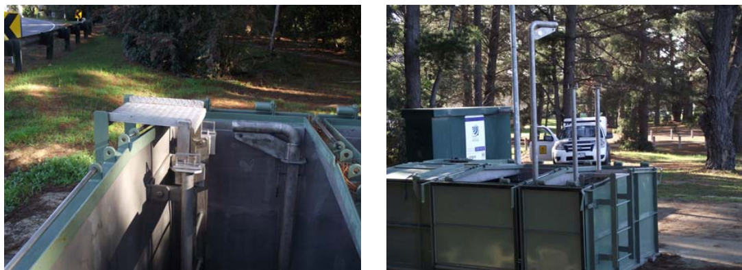
Figure 7: Ladder and davit arm positions for confined space entry, allowing other workers to operate safely on ground level, outside the opening.
