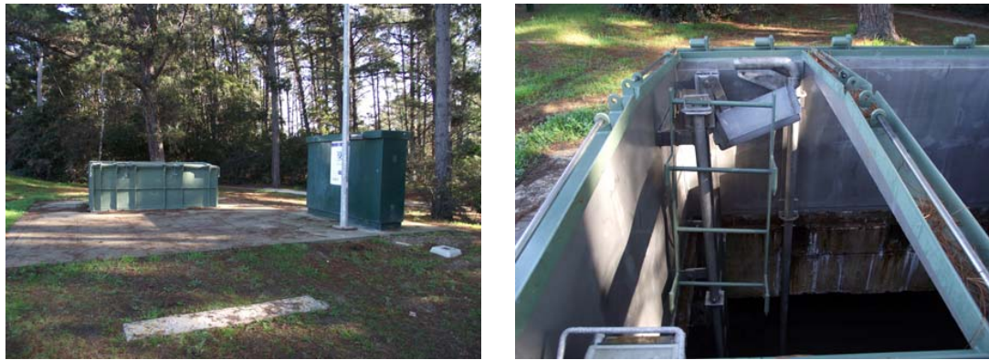
Figure 6: Turret with lid closed and then open, showing the ladder platform and davit arm folded down.
