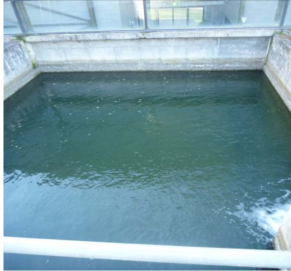
Figure 1: Maryborough WTP Filter
