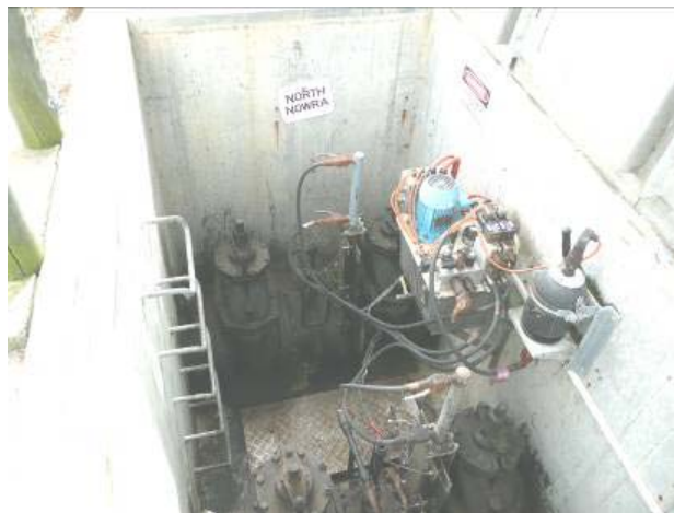
Figure 3: North Nowra surcharge main control valve
