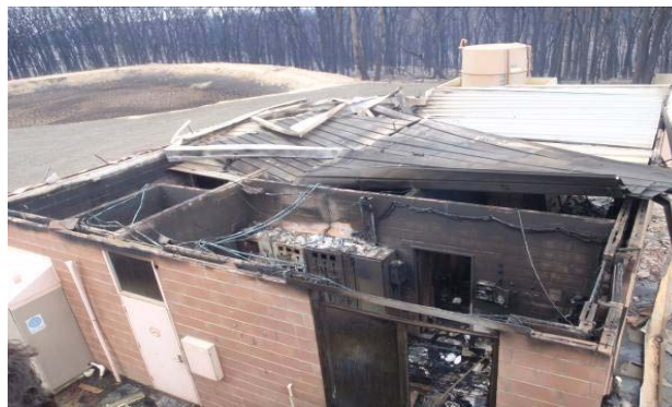
Figure 1: Burnt out dosing and control room
