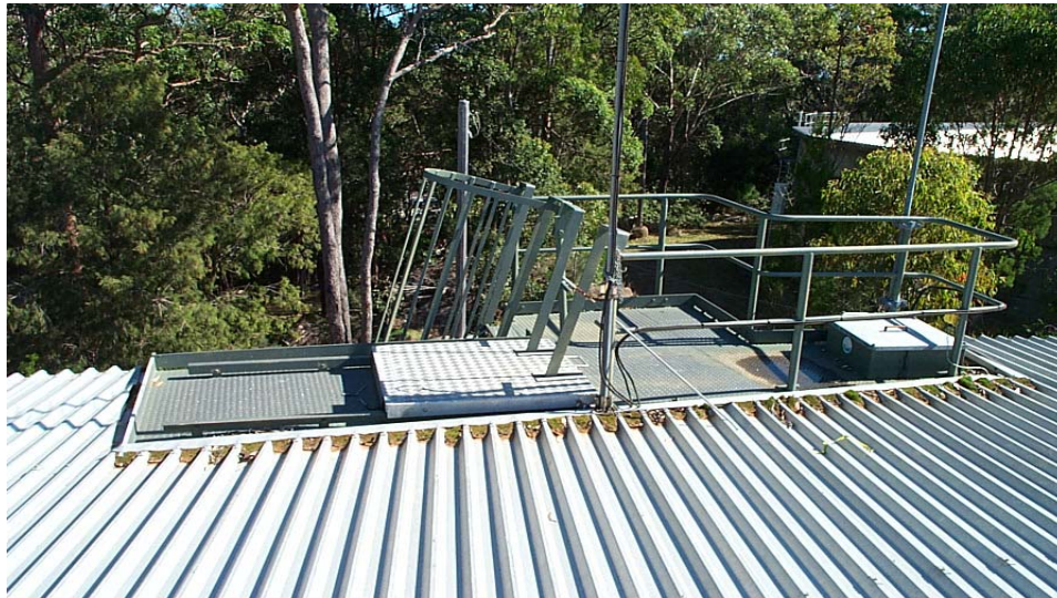
Figure 5: Typical platform area – roof debris is ponding, unsealed hatch area and lack of effective guard rails.
