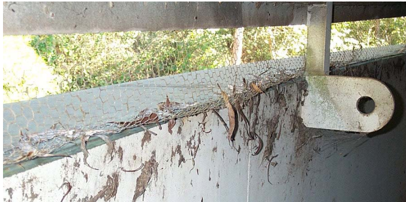
Figure 8: Ventilation mesh not effective against leaf debris & wind born contamination.
