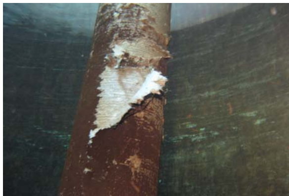
Figure 9: An AC overflow riser pipe that is de-laminating.
