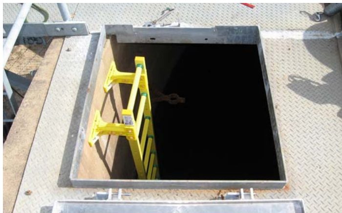
Figure 3: The hatch frame sealed off and a new vertical ladder fitted.
