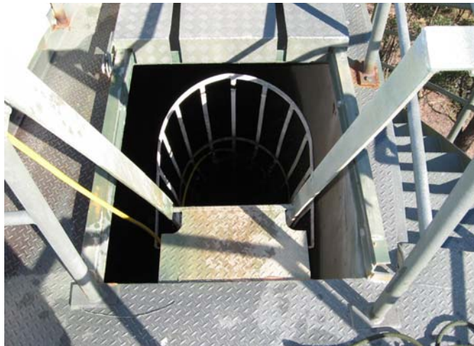
Figure 2: Ladder stiles protruding from an unsealed entry hatch area.
