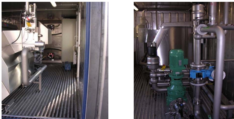
Figure 5: Tailored valves, feed pump, and optimized piping technology
