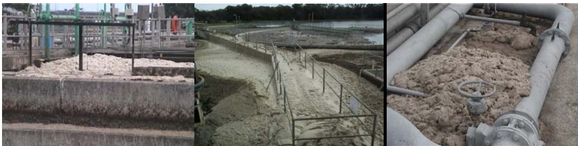
Figure 1: Examples of severe biological foaming at activated sludge plants.
