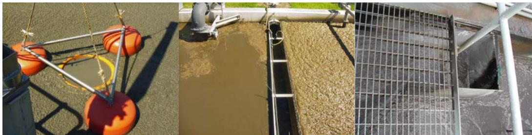
Figure 3: Trial bell mouth scum withdrawal, tipping scum pipe and surface waste activated sludge
