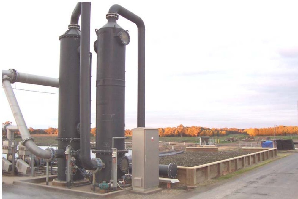
Figure 4: ATAD odour scrubbers at BWRP
