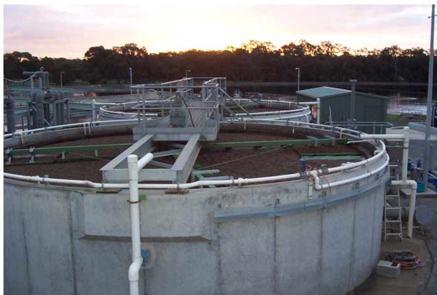
Figure 1: DAF thickened sludge
