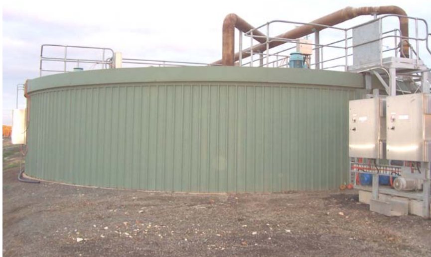
Figure 2: ATAD tank at BWRP
